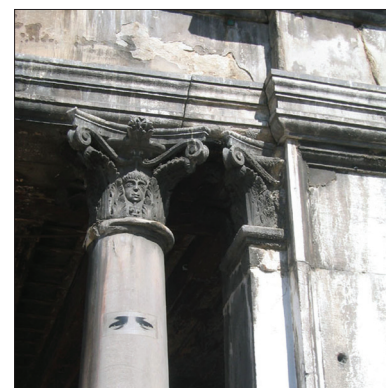
F4 Renovation of Clock tower in Piazza San Marco showing crack caused by a non-functional proposal
